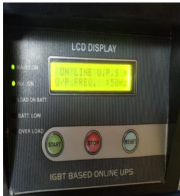
Fig.6. UPS is ON (On Battery Backup)
